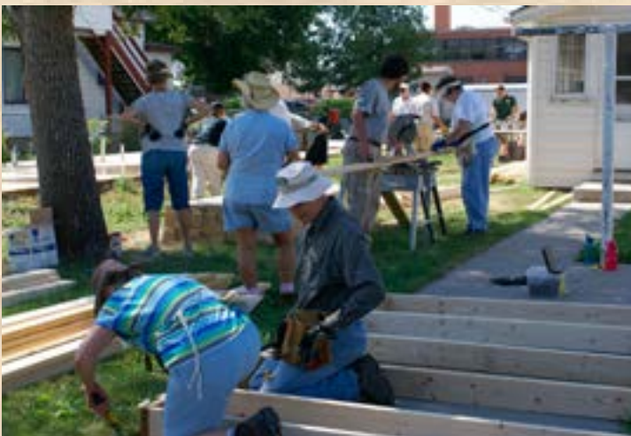
At least four smaller crews working on various aspects of the project. We used electric chop saws set up for working at waist height to cross-cut most of the dimensional lumber to the needed lengths.
