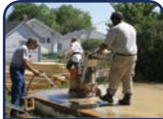
The author (with the hose working with an AmeriCorps volunteer from the Virgin Islands (running the concrete polisher).
