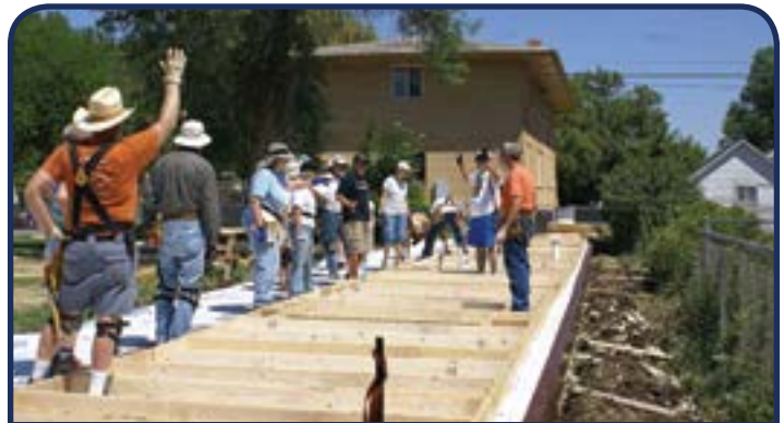
Getting ready to raise the east wall of the house. It is 76 feet long! You don't see that every day.
