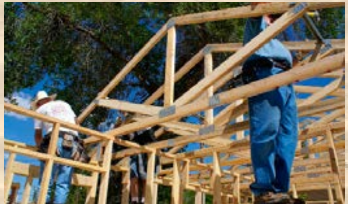
A 4-person crew from Colorado joined us for a day. Here they are securing trusses and bracing them with spacers.
