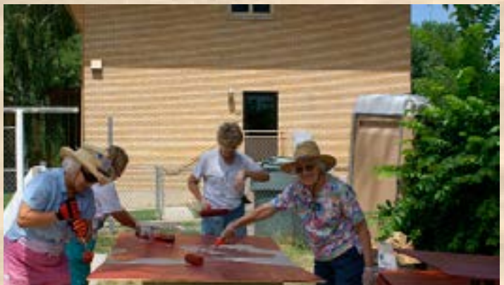
Another all-female group painting the siding. It was easier and more efficient to do this before it was installed as that allowed smaller teams to work in parallel without getting in each other's way.
