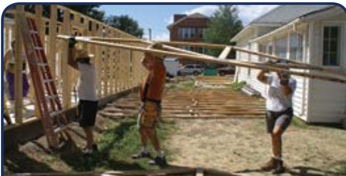
This is how we got the roof trusses up onto the roof; lift from below and pull from above. HFH builds are usually single story houses and rarely (if ever) use heavy equipment like cranes.
