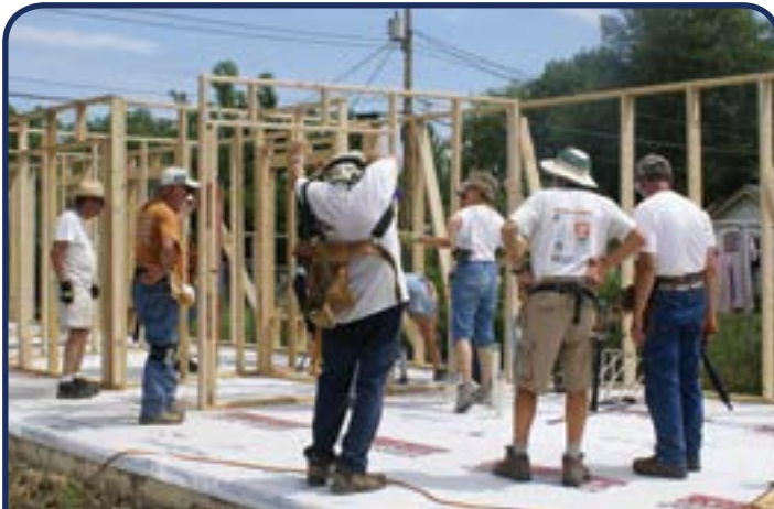
The house is starting to take shape. It was a thick slab-on-grade design with hot water radiant floor heat.
