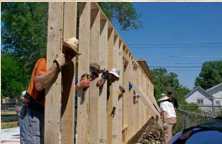
A few team members pose for a portrait as they hold the east wall in position while other team members secure the bracing.
