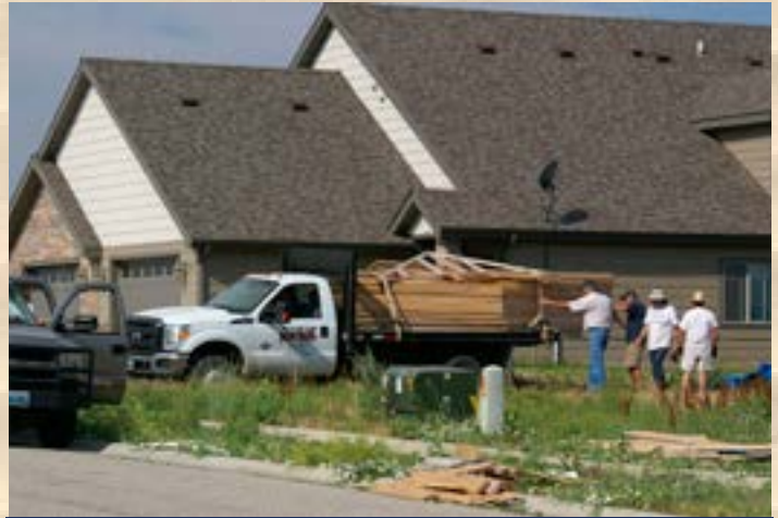
Picking up the roof trusses from another building site. (The house in the background is NOT an HFH home.)
