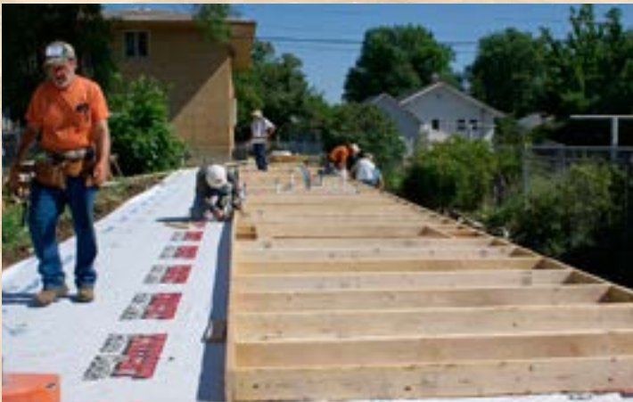
The east wall being worked on. You can see most of the 90 foot long foundation slab in this photo. Author is on the left (photo by Linda).
