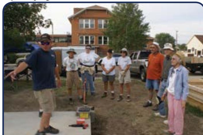
Part of our team at morning circle getting assignments for the day. Our HFH construction supervisor, Brian, apparently wants "it" over there.
