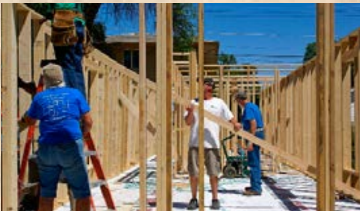
The west wall being braced. It was also 76 feet long and built as a single unit before standing it up. This is a "shotgun" house, 14 feet wide and 76 feet long not including the front porch.
