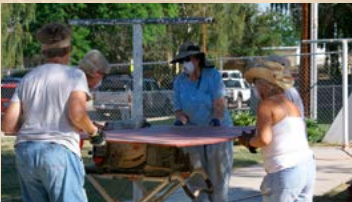
An all-female crew running sheets of siding plywood through the table saw. Two of the women in this group were singles. HFH builds are not just for RVing couples.
