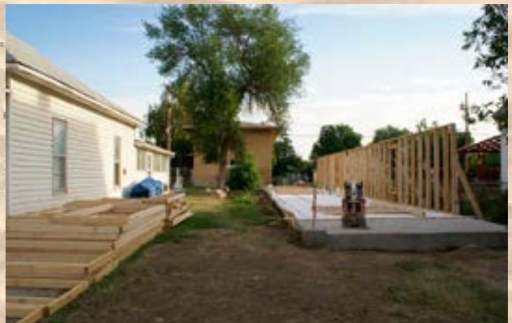
The building site after erecting the east wall. The photo clearly shows the foundation slab. Partition walls are stacked to the left.
