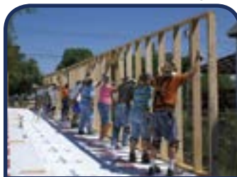
The east wall standing up. We had to hold it until it was braced.
