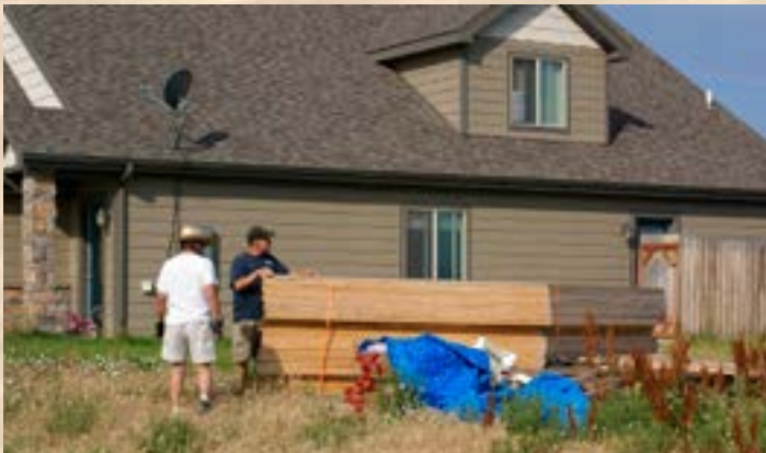
This is how the roof trusses were delivered to the other site. We had to un-band them and load them onto a flatbed truck one at a time.
