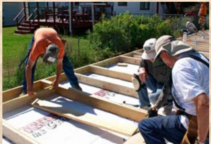
Framing in an opening for a window in the 76 foot long east wall.
