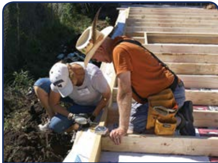
A husband and wife team working on the east wall of the house.
