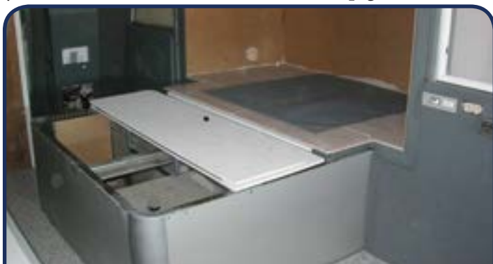
Instant water heater cabinet
