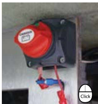
Battery disconnect switch used to turn FPM-50 on/off
