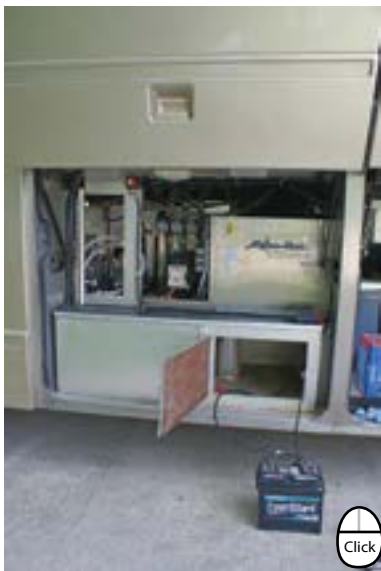
The Aqua-Hot is center right. The FPM-50 is in the small vertical compartment center left. The battery for the FPM-50 will go in the compartment below the Aqua-Hot.
