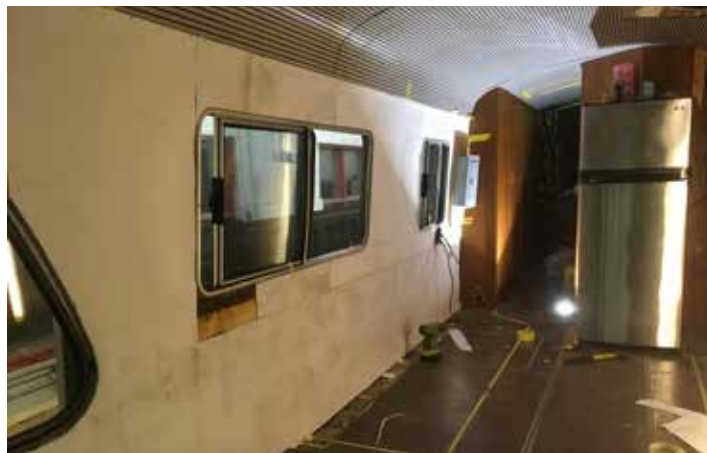
Insulation and wall covering done, ready for the first trip with a well insulated coach.
