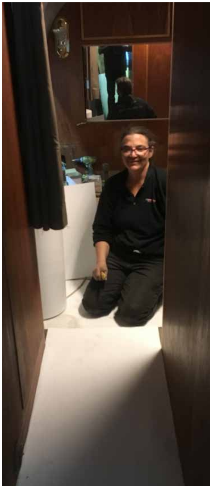
EHP being installed on the hall and bedroom floor by the lady of the house.
