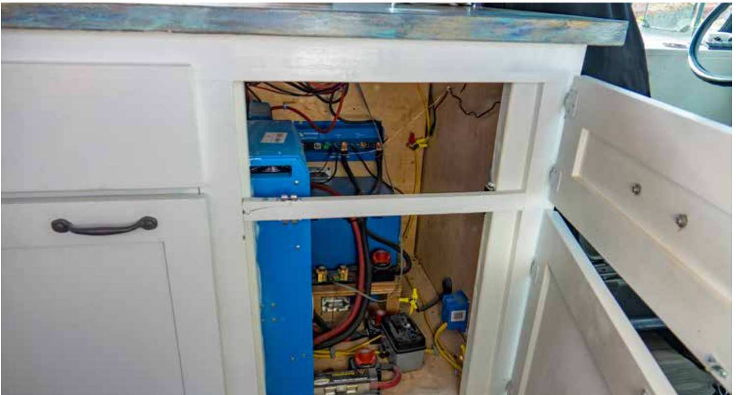
Our Power System.
